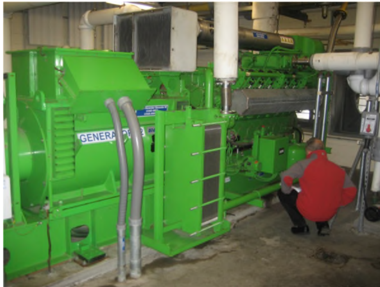
Figure 1: Example of Reciprocating Engine Powered by Biogas Source: Tetra Tech
